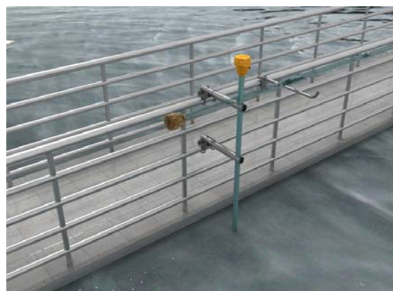
pH/ORP reaction pool installation
